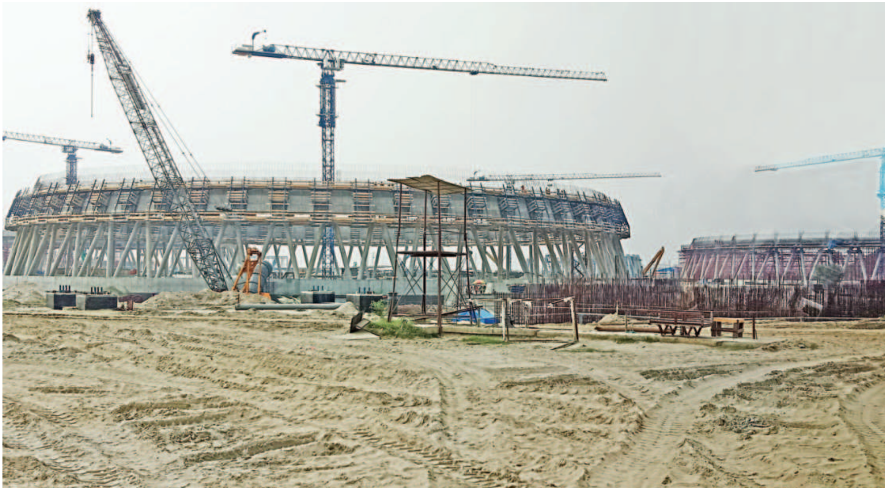
The construction of the cooling unit, one of the major components of the Rooppur Nuclear Power Plant in Pabna, is underway. Russia is providing Tk 91,040 crore for the Tk 113,092 crore project, which is expected to become operational in 2023. The photo was taken on October 10 last year.
