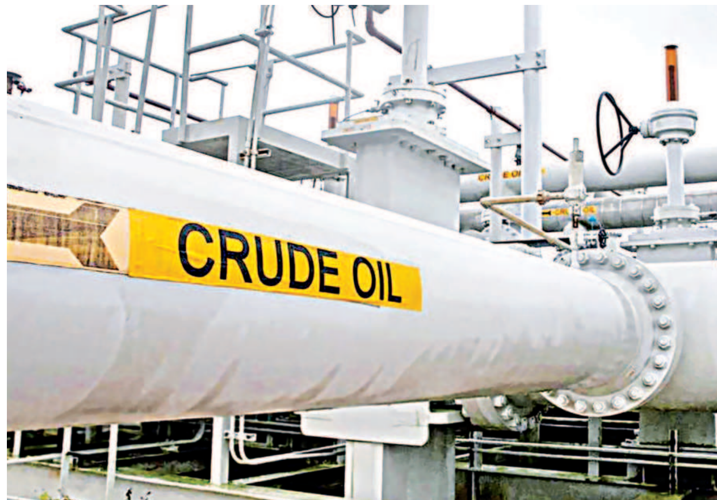
A maze of crude oil pipes and valves is pictured during a tour by the Department of Energy at the Strategic Petroleum Reserve in Freeport, Texas.
