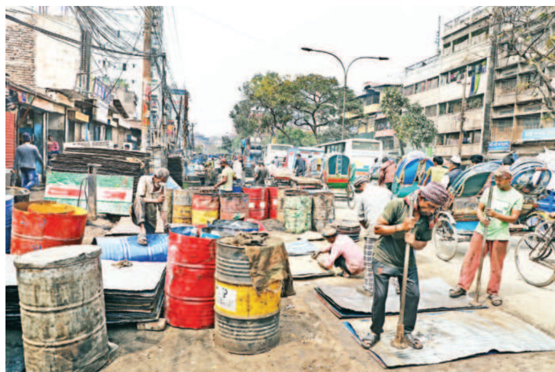
Leaving a narrow width for vehicular movement, a busy road in the capital's Dholaikhal is being mended by authorities. On the left, the footpath has been taken over with large drums of asphalt, obstructing pedestrian movement and putting them at risk as they try to cross the space. Although meant to benefit commuters, the reconstruction, in hindsight has led to more peril for citizens. This photo was taken yesterday.
