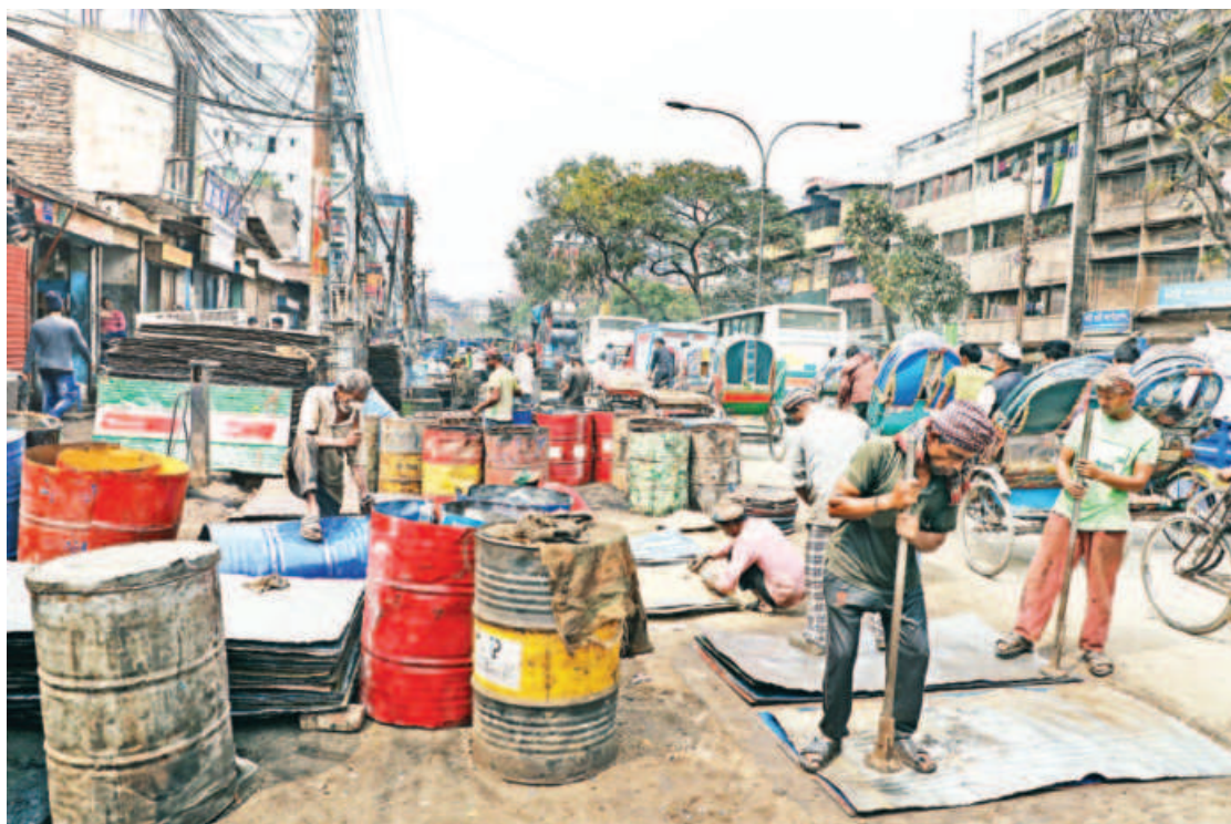
Leaving a narrow width for vehicular movement, a busy road in the capital's Dholaihal is being mended by authorities. On the left, the footpath has been taken over with large drums of asphalt, obstructing pedestrian movement and putting them at risk as they try to cross the space. Although meant to benefit commuters, the reconstruction, in hindsight has led to more peril for citizens. This photo was taken yesterday.
