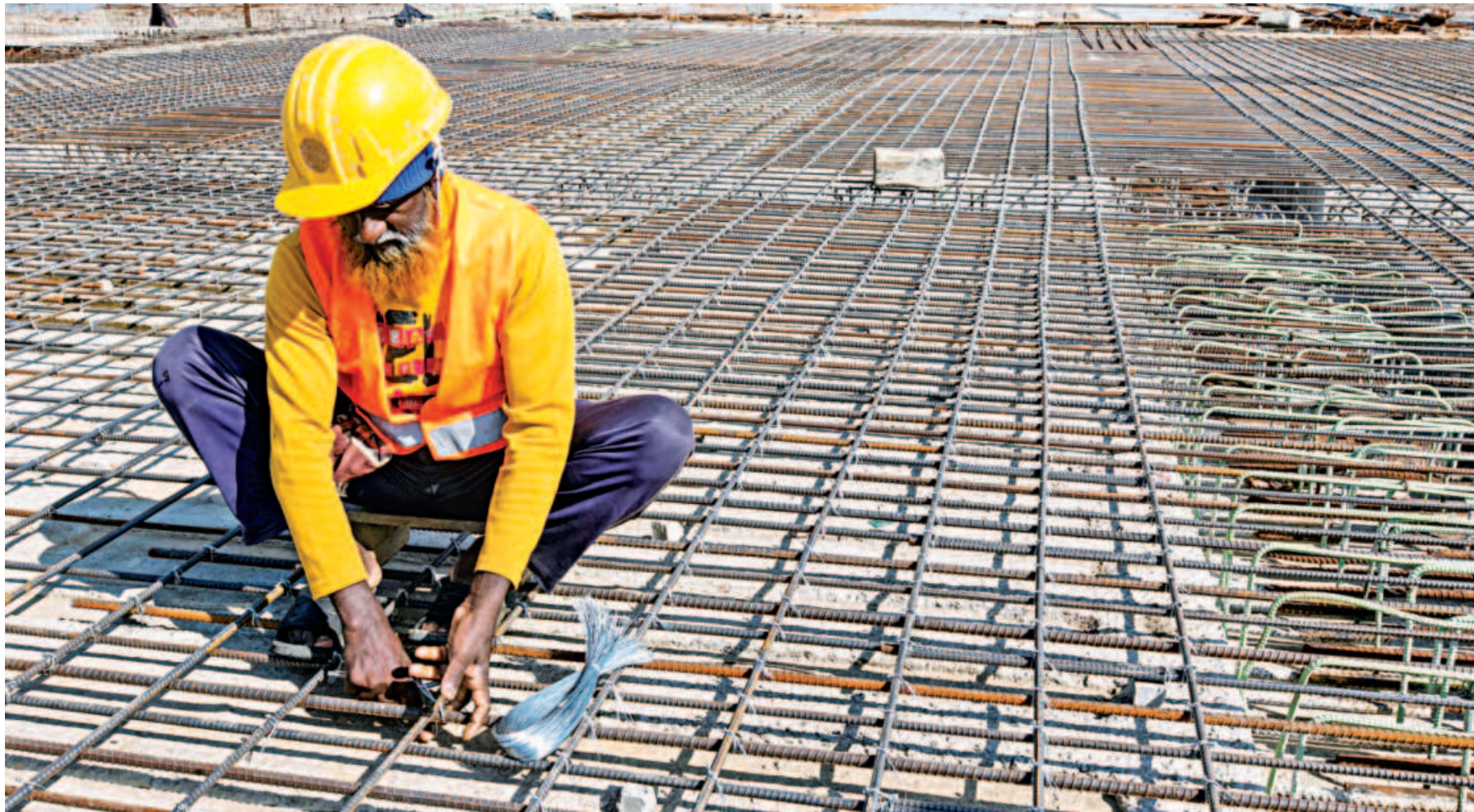
A worker binds steel rods at the under-construction Patenga Container Terminal of the Chattogram port. Steel prices have jumped 19 per cent over the past one year. Mild steel (MS) rod (60 grade) sold for Tk 82,500 per tonne yesterday, according to the Trading Corporation of Bangladesh. The photo was taken earlier this month.
