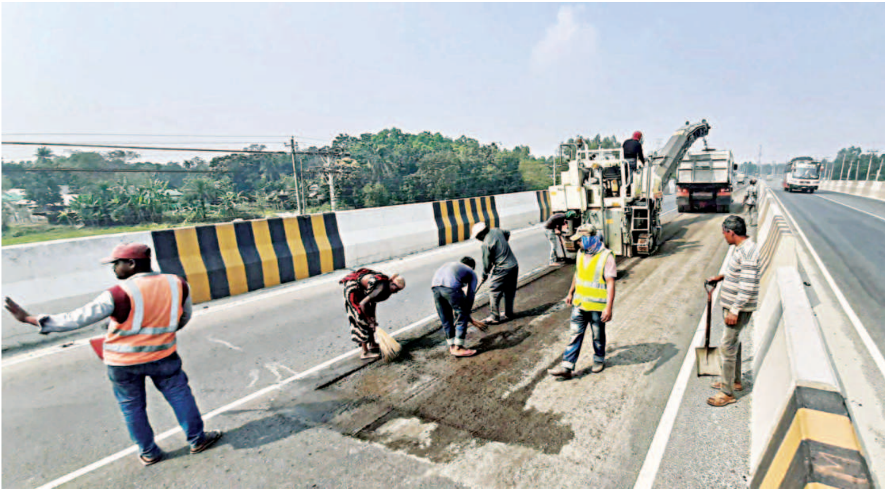
Workers are carrying out last-stage tasks of the long-awaited Joydevpur-Elenga Highway project as the initiative is set to complete by December this year. Finally, the project cost might stand at Tk 6,168 crore.
