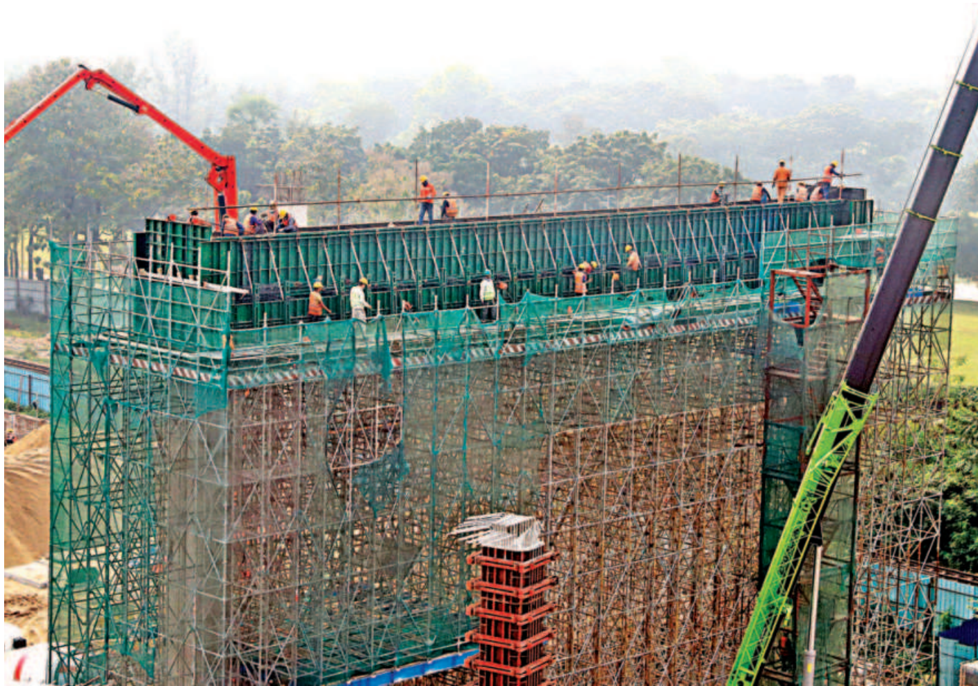
Construction workers engaged in the Banani section of the 19.73-kilometre Dhaka elevated expressway. The project is scheduled to be completed in June 2023.
