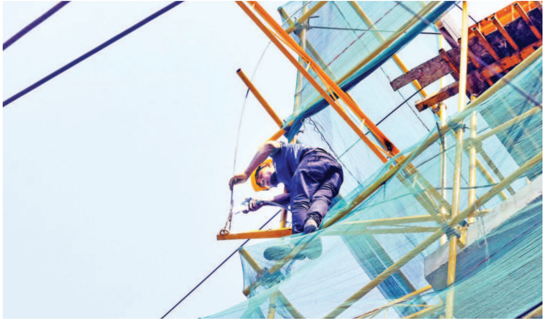
A worker risking his life while working on a multistorey under-construction building in the capital's Jigatola area. The authorities concerned remain oblivious to the dire consequences of the lack of safety measures. The photo was taken yesterday.
