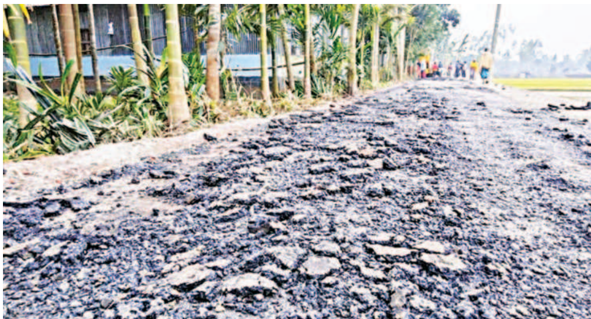
The newly completed carpeting of a paved road in Ulipur upazila of Kurigram got damaged, bearing testimony to the low quality work. PHOTO: COLLECTED
