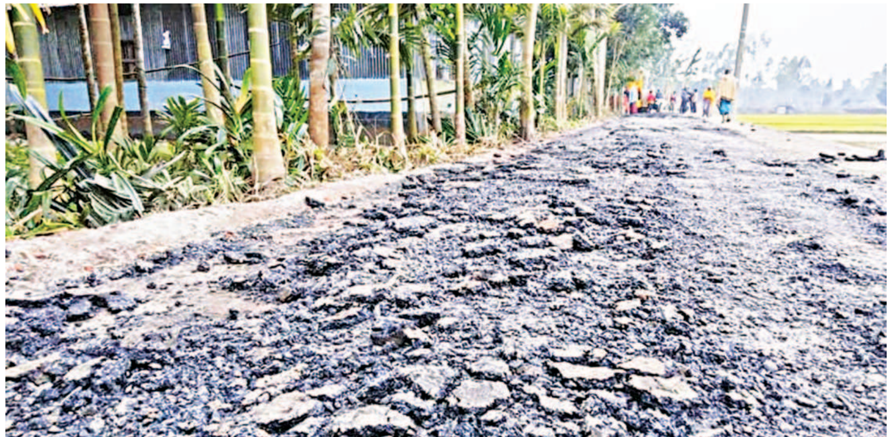
The newly completed carpeting of a paved road in Ulipur upazila of Kurigram got damaged, bearing testimony to the low quality work.
