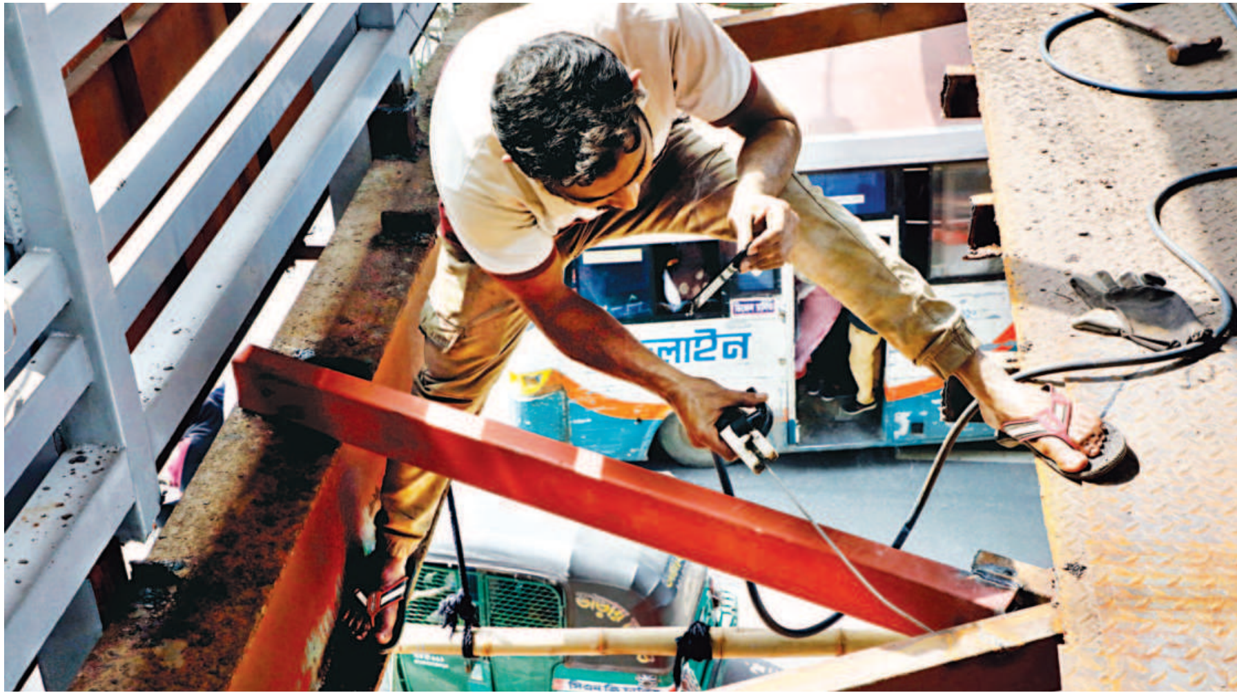
With no safety gear on, a worker welds a gaping hole on a foot-over bridge on the busy Satmasjid Road. Right through the hole, vehicles can be seen passing by the highly hazardous working environment. At any point, either workers or commuters can fall victim to a dangerous accident. This photo was taken yesterday.
