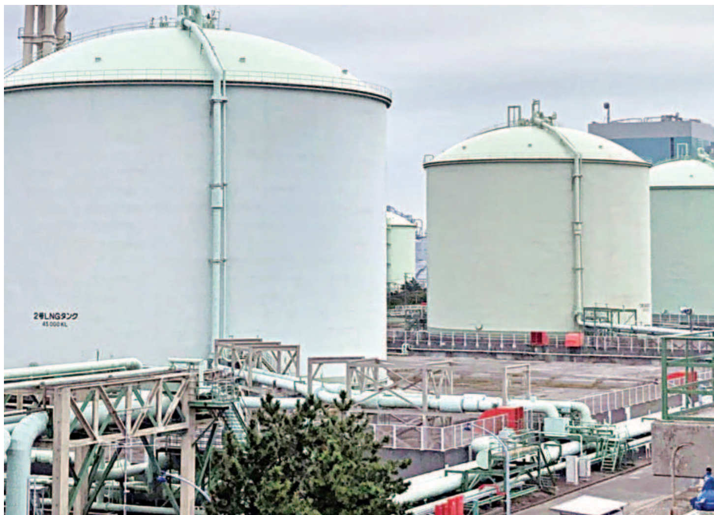
A general view of the Negishi LNG Terminal which is jointly operated by Tokyo Gas and JERA in Yokohama.
