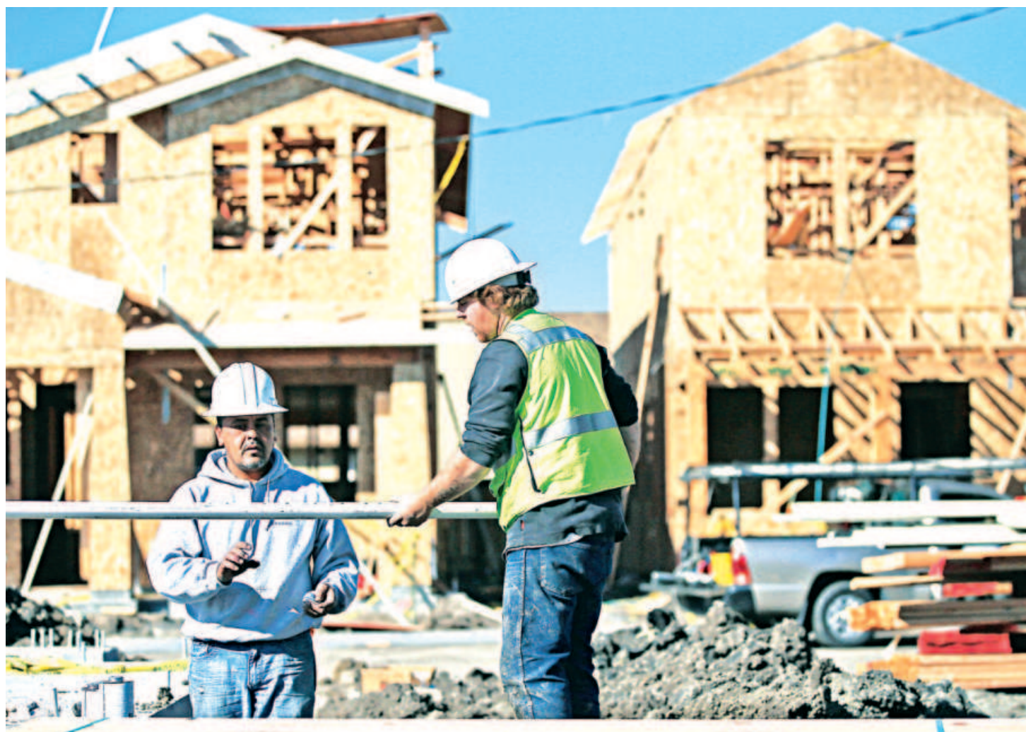
Workers prepare to move a piece of pipe into place as they build a new home in Petaluma, California.
