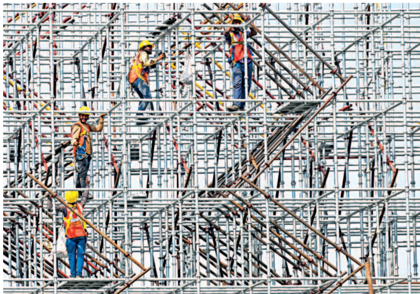
Labourers work at a coastal road construction site in Mumbai, India on January 12. Asia's third largest economy has been on the mend after the government lifted mobility measures.
