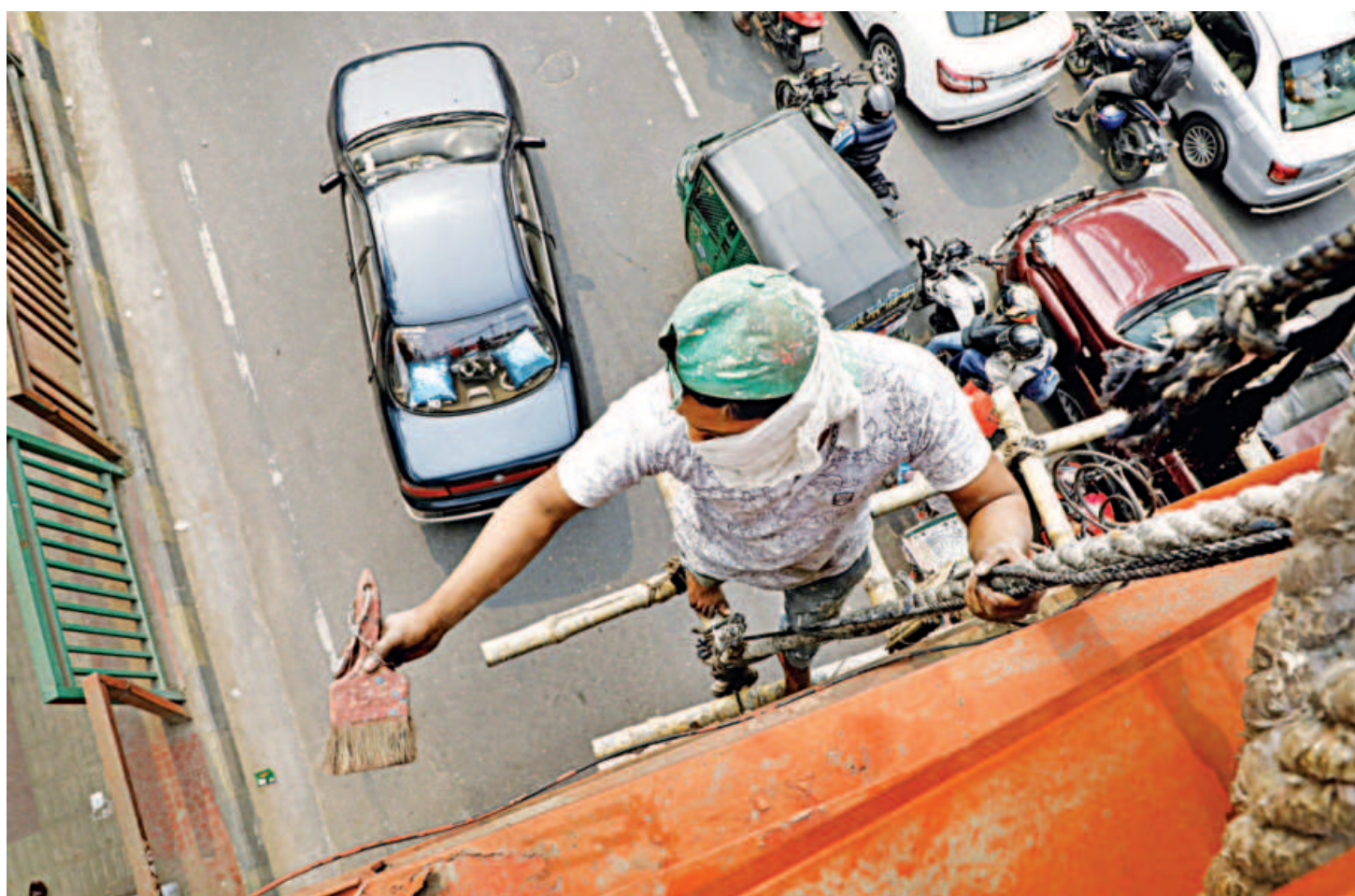
Grasping a rope with one hand, a man paints a footbridge with the other while standing on some rickety bamboo poles tied together in Science Laboratory area of the capital yesterday. He had no safety harness and could have fallen to his death or injured himself. Many workers put their lives at risk every day for wages on which their families can hardly survive.
