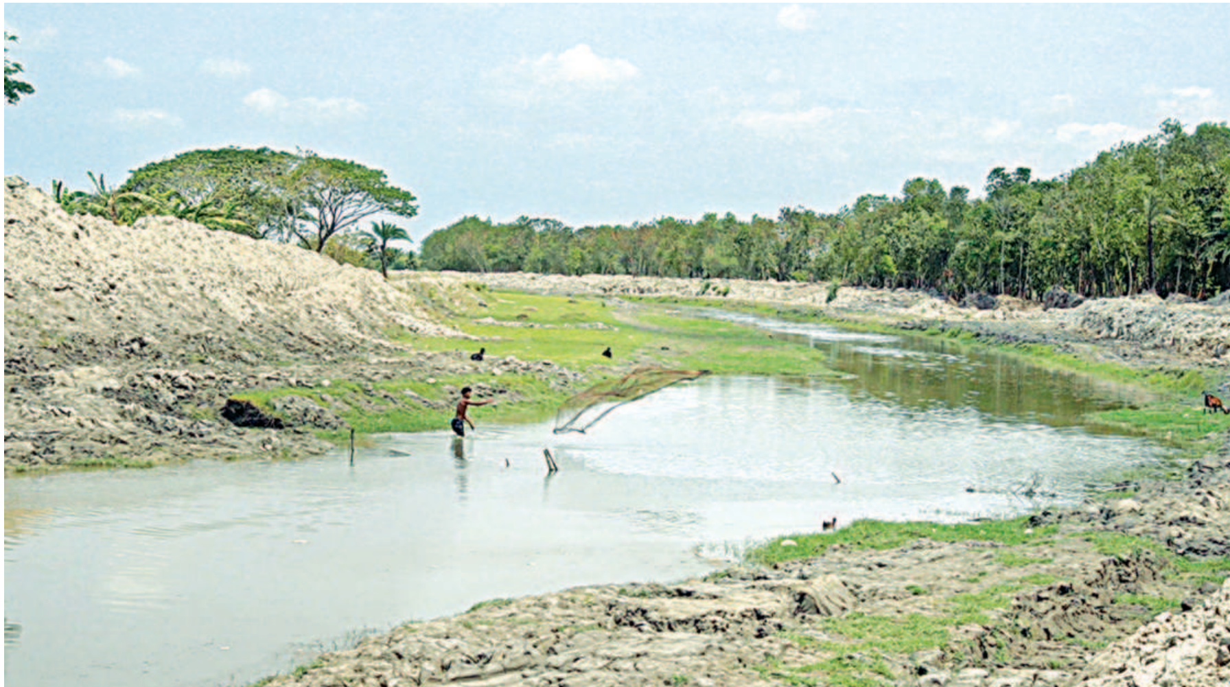
The never-ending Bhabadah waterlogging saga continues, with stories of negligence, mismanagement and even alleged corruption piling up. Beyond just people of the area, rivers such as Teka and Hari are victims to the whole situation as well. As excavated earth is dumped back onto them, both of the rivers suffer from siltation, which is raising the riverbed as well as choking the rivers' width.
