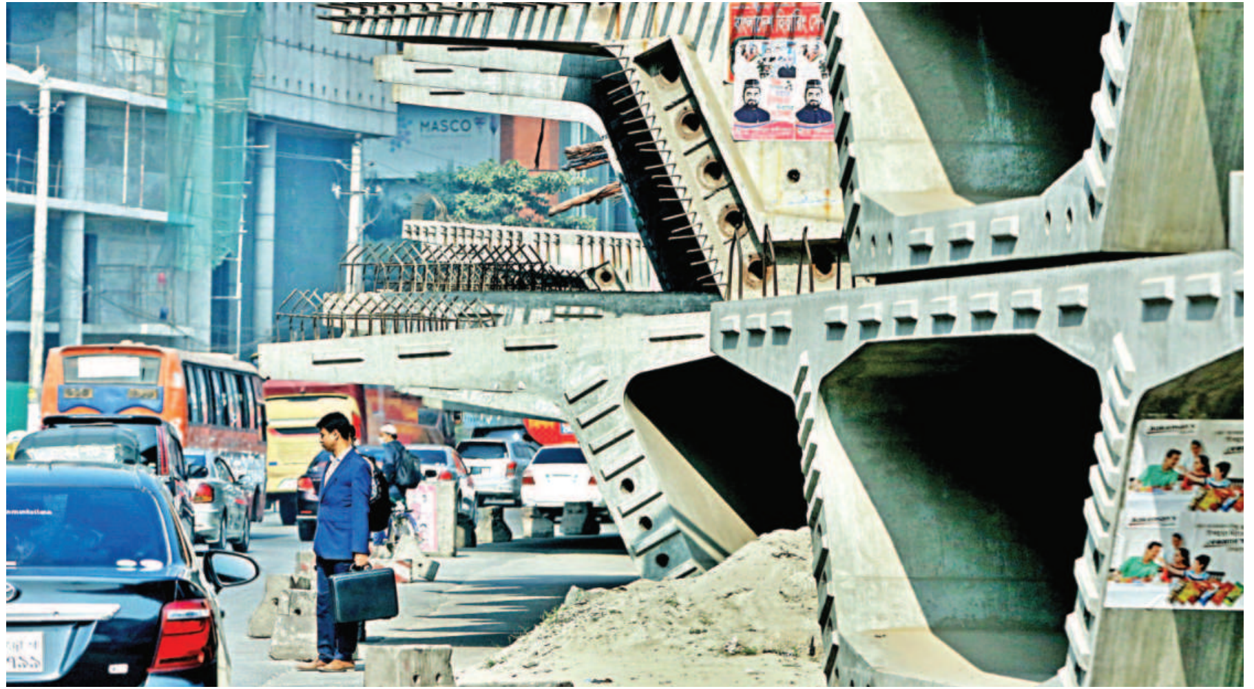
These girders are supposed to be used for the Bus Rapid Transit project. But for the last year and a half, they've been left lying there on Airport Road. Their presence chokes the critical road, which is a gateway for inter-district vehicles, and leads to chronic traffic jams in the area. This photo was taken near the airport yesterday.
