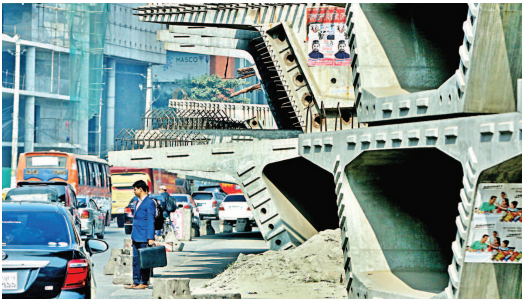
These girders are supposed to be used for a mega project. But for the last year and a half, they've been left lying there on Airport Road. Their presence chokes the critical road, which is a gateway for inter-district vehicles, and leads to chronic traffic jams in the area. This photo was taken near the airport yesterday. PHOTO: ANISUR RAHMAN
