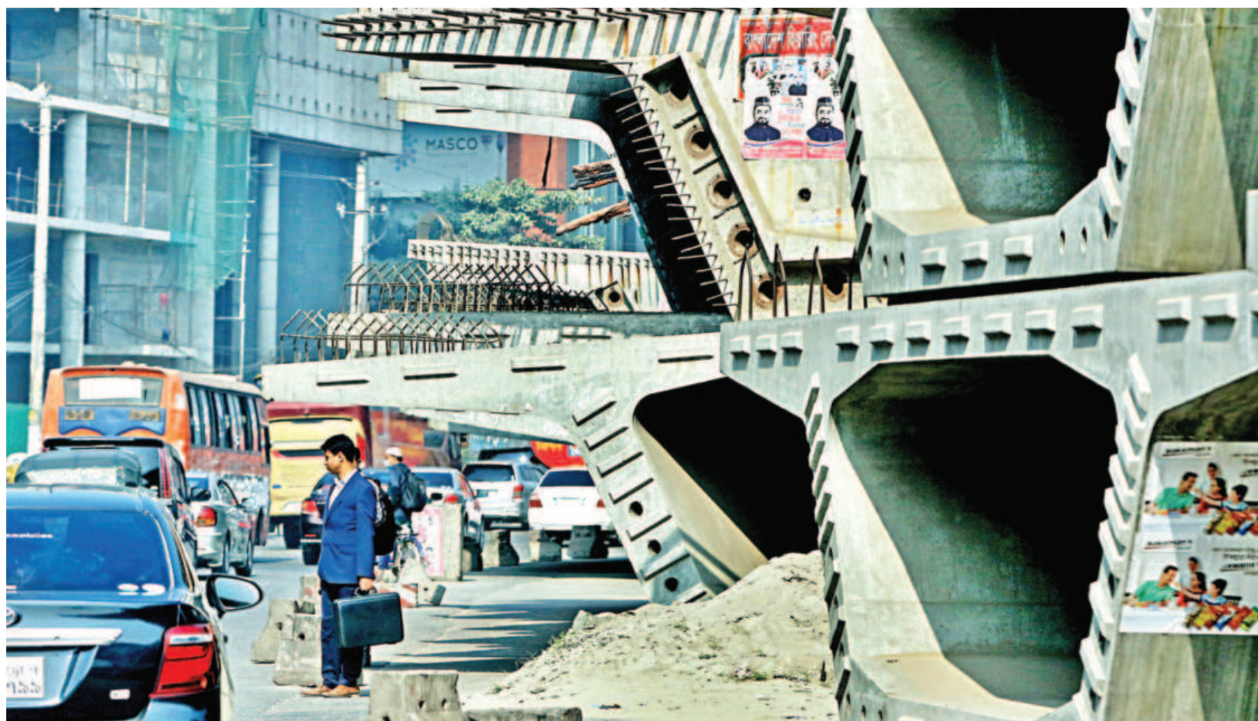
These girders are supposed to be used for a mega project. But for the last year and a half, they've been left lying there on Airport Road. Their presence chokes the critical road, which is a gateway for inter-district vehicles, and leads to chronic traffic jams in the area. This photo was taken near the airport yesterday. PHOTO: ANISUR RAHMAN
