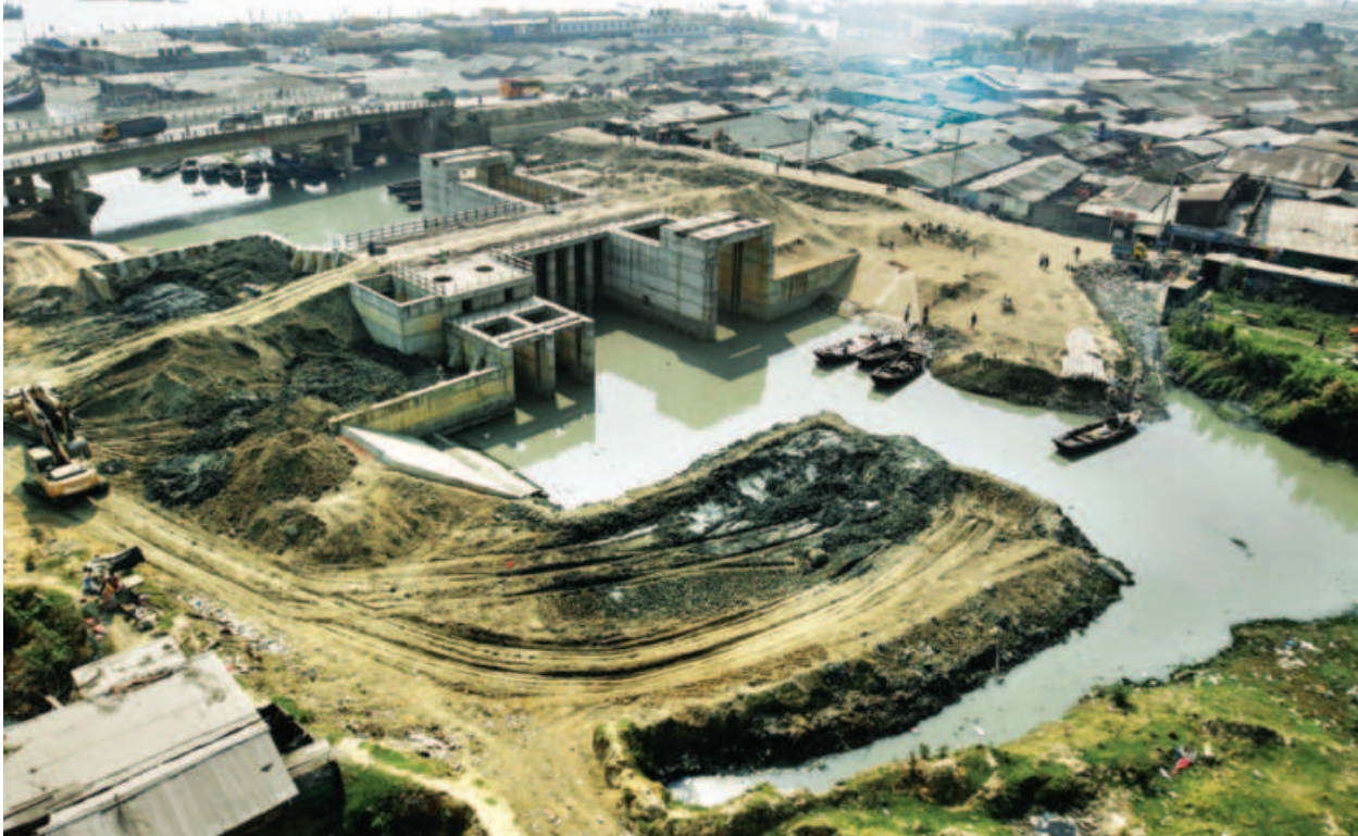
A sluice gate being installed at the mouth of the Rajarkhali canal on the bank of the Karnaphuli in Chattogram. To lessen the impacts of waterlogging, various local organisations are installing around 40 such sluice gates at points where canals in the port city fall into the river. The photo was taken yesterday morning.
