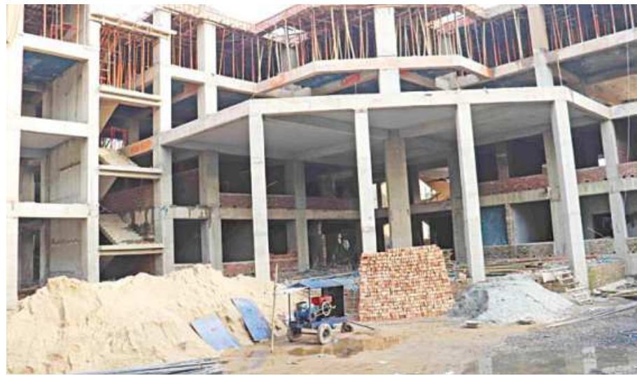
The construction work of 250-bed hospital in Pirojpur town progresses in full swing.
