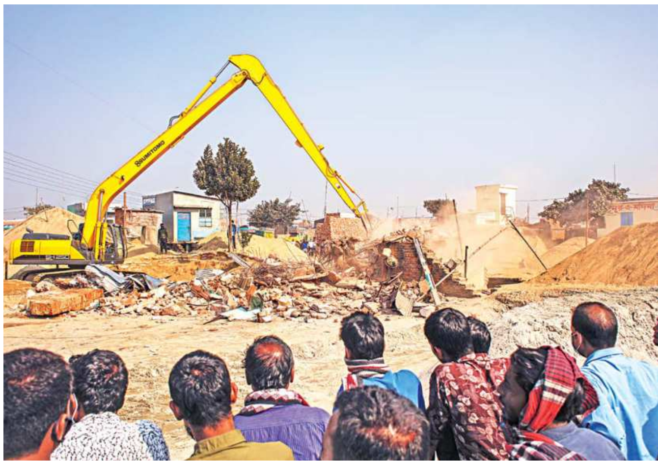
Bangladesh Inland Water Transport Authority yesterday demolished illegal structures at Koyla Patti area in the capital's Gabtoli.
