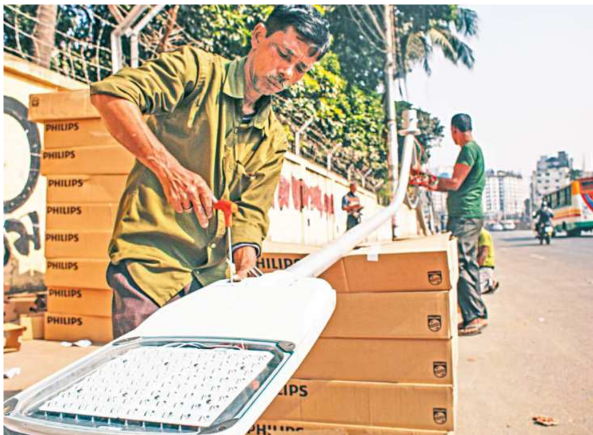
Dhaka North City Corporation is installing energy efficient LED street lights at different areas under its jurisdiction. Many roads of the capital are dimly lit, and the move aims to help drivers and pedestrians after sundown. This photo was taken from Kalyanpur area yesterday.
