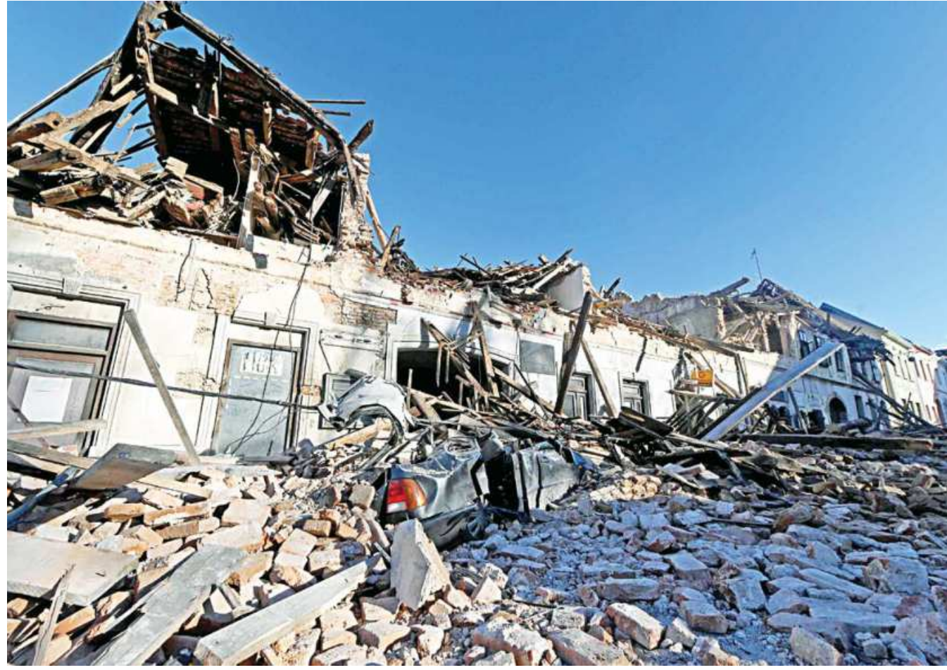
The wreckage of a car and damaged buildings are seen in Petrinja, some 50kms from Zagreb, after the town was hit by an earthquake of the magnitude of 6.4.
