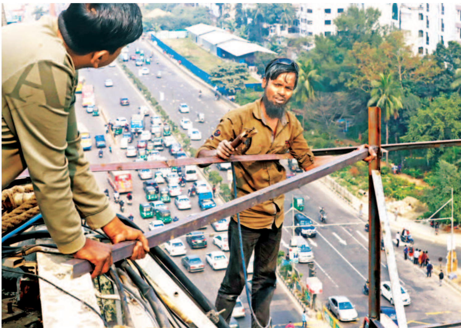
Two men are repairing a billboard at Chairmanbari in the capital's Banani area yesterday. They neither have any safety gears nor any safety harness. A little slip and a tumble from that height could be fatal.
