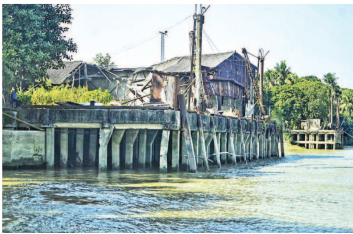
A partly collapsed structure of the state-owned Khulna Newsprint Mills on the Bhairab river in the southwest of Khulna city. The mill has been shut for two decades as it incurred heavy losses after the demand for its newsprint decreased. However, the authorities are still paying different bills of over Tk 14 lakh a month. The photo was taken recently.
