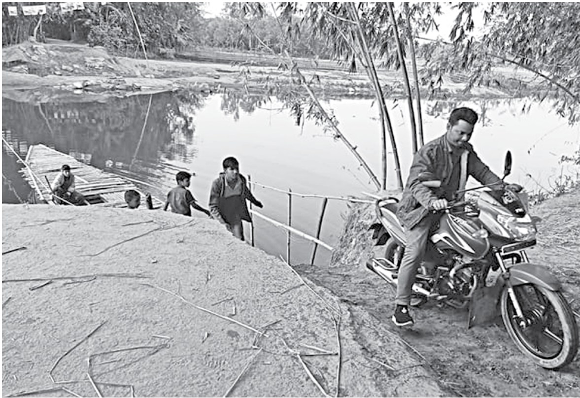
The collapse of a boat ghat on Gaddimari-Barakhata road at Niz Gaddimari village of Hatibandha upazila in Lalmonirhat causing untold sufferings to the residents of six villages.
