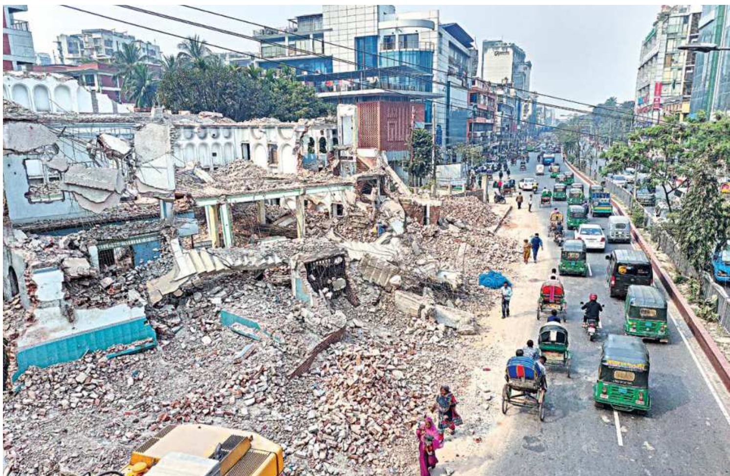
In the quest for reconstructing the Dhanmondi Sobhanbagh Mosque, the old structure has been demolished recently. Laden right onto the open road, with no fences in place to contain the rubble, the deconstructed site poses safety concerns for commuters using the busy street. This photo was taken yesterday.
