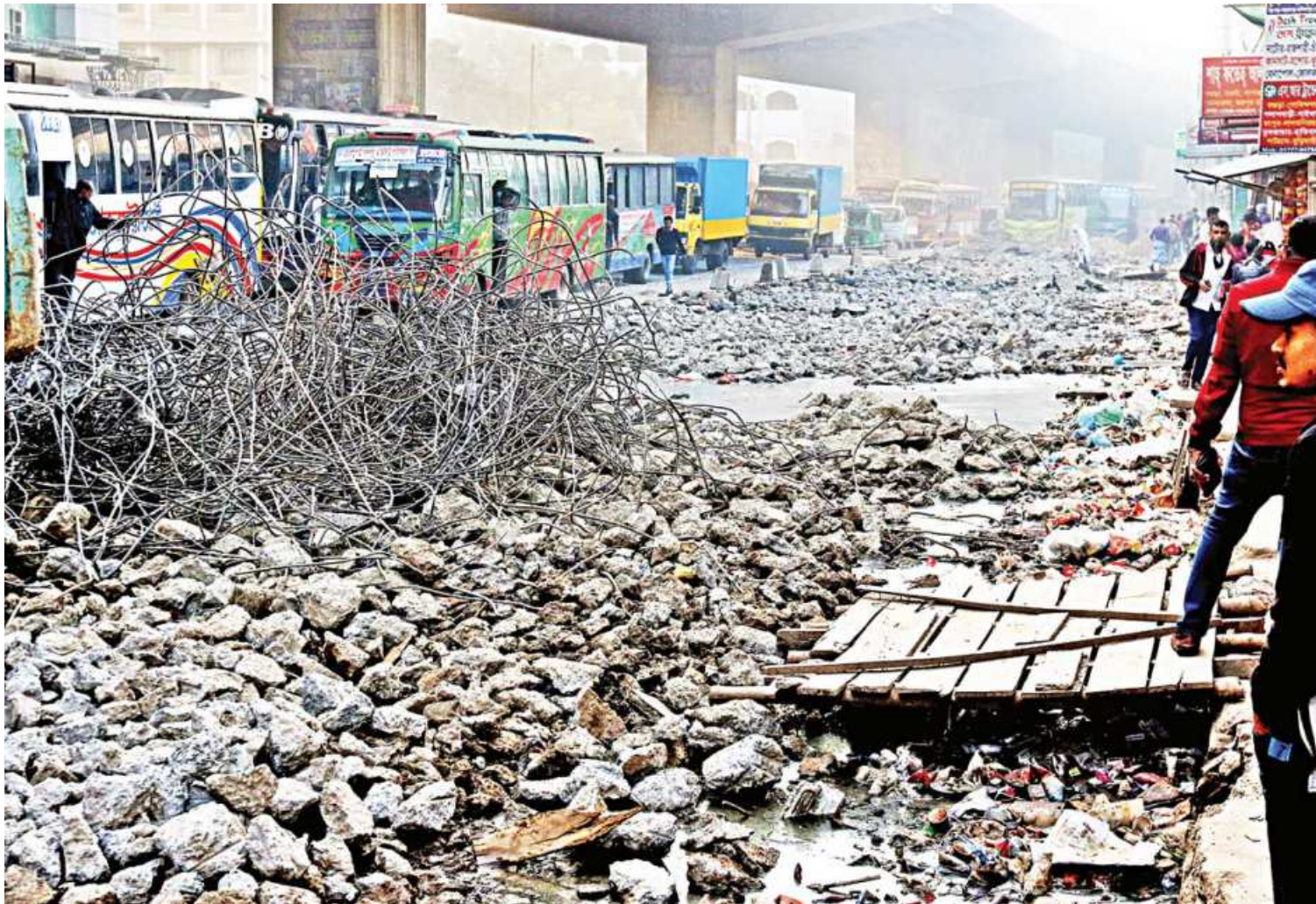
For the construction of lanes for Bus Rapid Transit, this section of the Dhaka-Mymensingh highway in Azampur of Uttara has been dug up and left like this. There seems to be inadequate warnings and protection for motorists and pedestrians using the highway.
