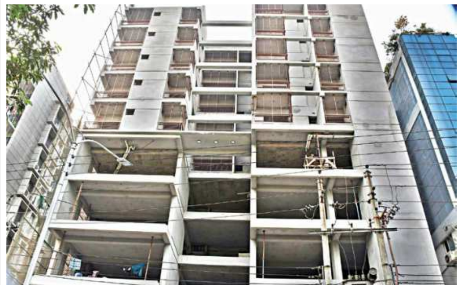
If the housing sector moves forward, so too will backward linkage industries such as cement, paint, steel and ceramics, said Alamgir Shamsul Al-Amin, president of REHAB.
