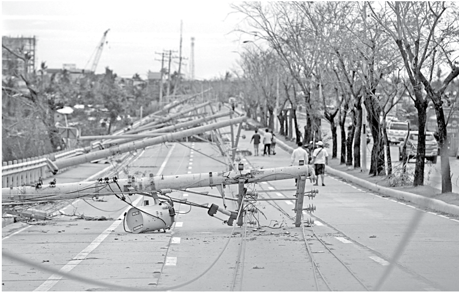
Residents walk past downed electric pylons in Talisay town, Cebu province yesterday, a day after Super Typhoon Rai pummelled the southern and central regions of the Philippines. At least 12 people have died in the strongest typhoon to hit the Philippines this year, the disaster agency said.
