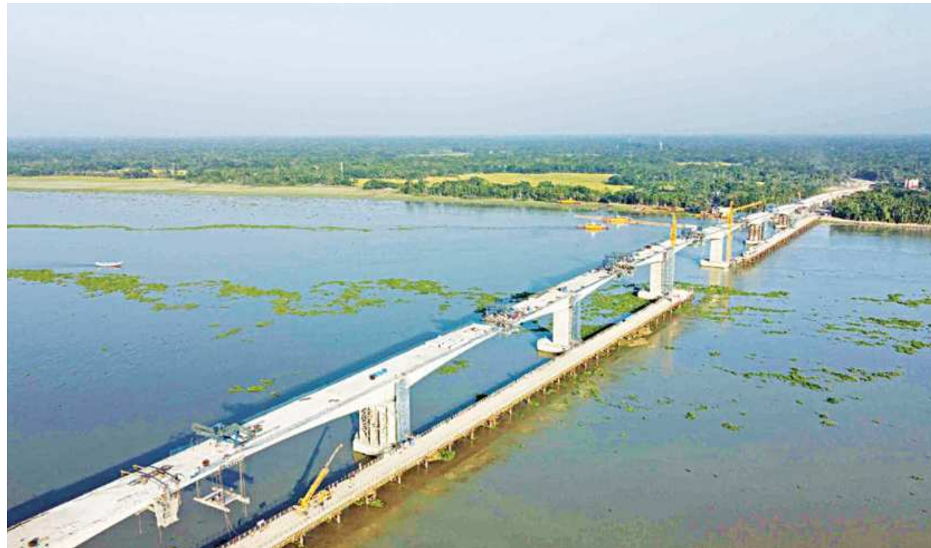
An aerial view of the eighth Bangladesh-China Friendship Bridge on the Kacha river in Pirojpur. The bridge project is supposed to be completed in June 2022.
