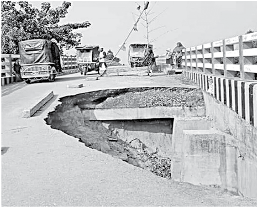
Plying of heavy or medium vehicles remains snapped since a large portion of this bridge, on Naaldiga river in Netrakona's Kalmakanda upazila, collapsed a few weeks ago.
