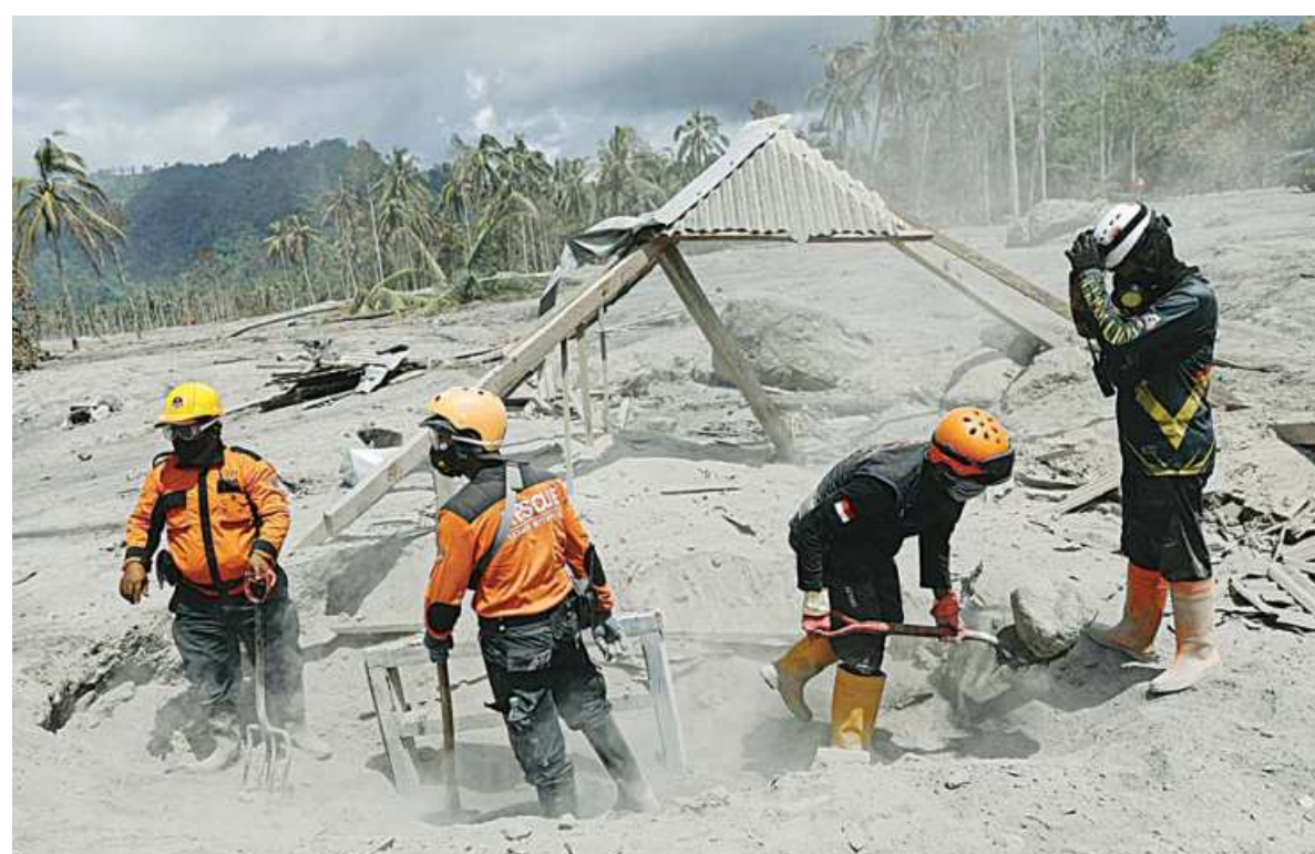
Rescuers dig a damaged building during an operation at an area yesterday which was affected by the Mount Semeru volcano eruption that killed at least 43 people last Saturday in Sumberwuluh, Candipuro district, Lumajang, East Java province, Indonesia.
