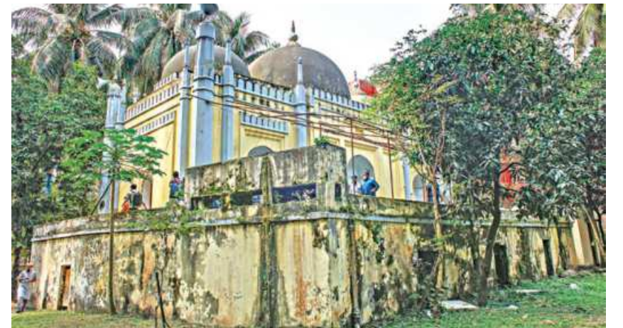
Prayers are still offered at the Musa Khan Jame Mosque, but its ailing state, due to lack of preservation, disappoints history enthusiasts. Fifteen other historic sites on the Dhaka University premises suffer similar conditions. The photo was taken recently.
