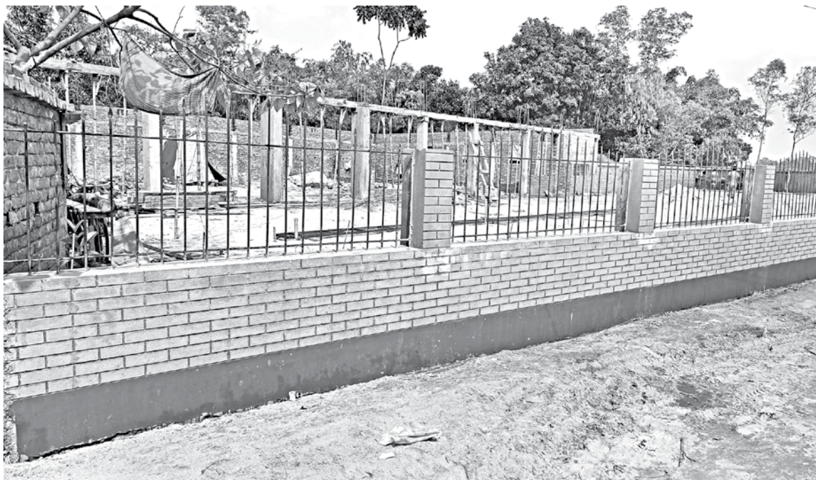
A view of the illegal structure built on the land of the Water Development Board along the flood bypass road next to the Teesta Barrage in Doani area of Lalmonirhat's Hatibandha. A local Awami League leader claimed that he was building the structure on his own land but failed to show any document in favour of his claim. PHOTO: STAR
