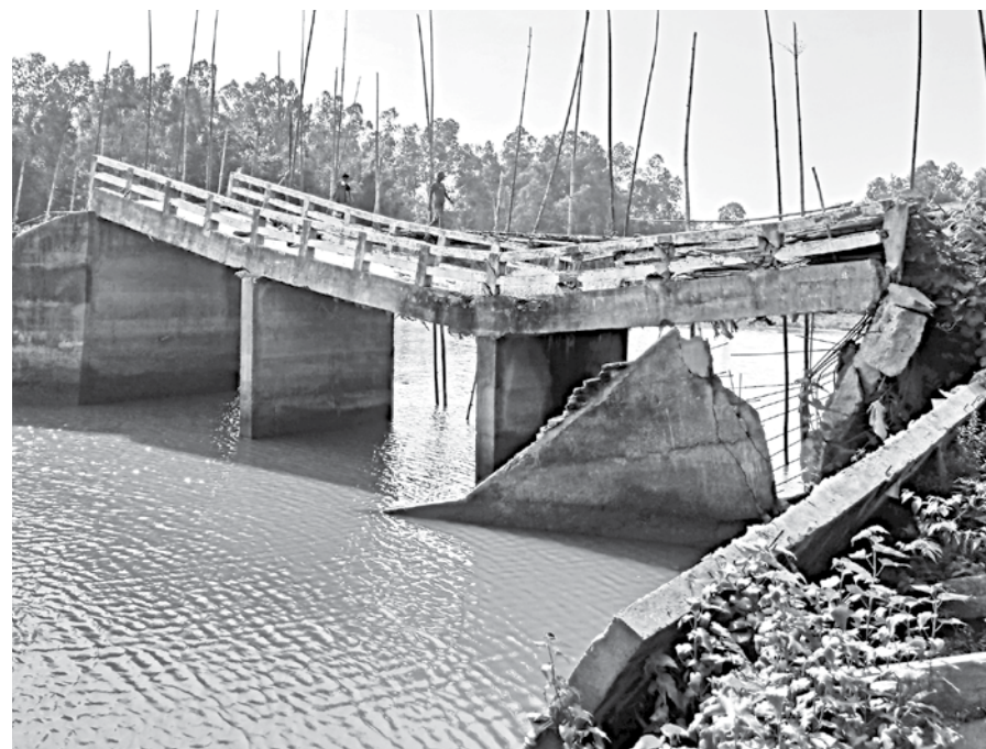
This bridge over a canal at Charshoulmari Bazar in Kurigram's Roumari upazila collapses only over a year of its construction, causing immense suffering to the locals.
