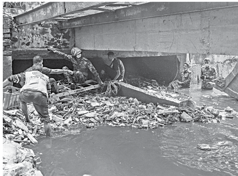
Fire service personnel rummage through the waste-filled waters of the drain yesterday, where Kamal went missing on Monday. PHOTO: RAJIB RAIHAN
