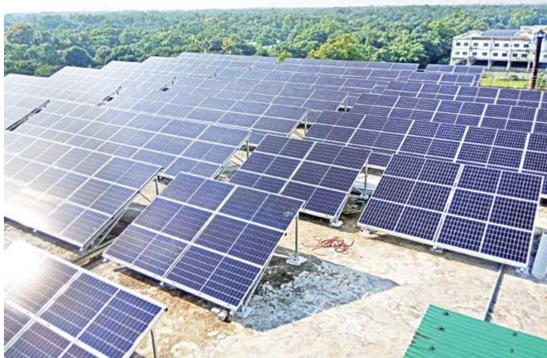
Industrial rooftop solar power projects could be a significant contributor to the country's energy grid as it is cheaper and cleaner to produce electricity from renewable sources such as this compared to traditional methods.
