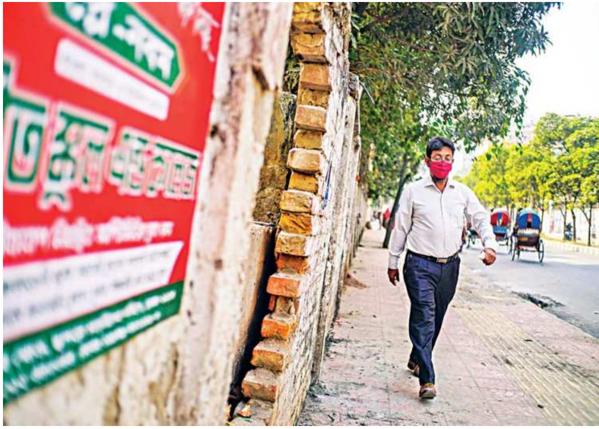
Although Tuesday's accident at Azimpur -- which killed schoolboy Zihad Hossain after a wall collapsed on him -- captured the public's attention, this has been a long-standing problem all across the city. For example, right beside Azimpur at Palashi Residential Area, there are similar tilted walls, which might collapse anytime and spell disaster for unsuspecting pedestrians. This photo was taken yesterday.
