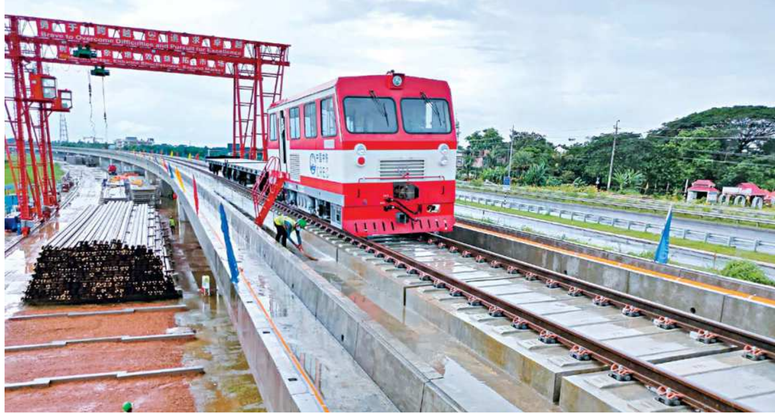
A view of the Padma bridge rail link project at the Mawa end in Munshiganj. Contractors of infrastructure projects have demanded that the government raise the procurement prices of construction materials.
