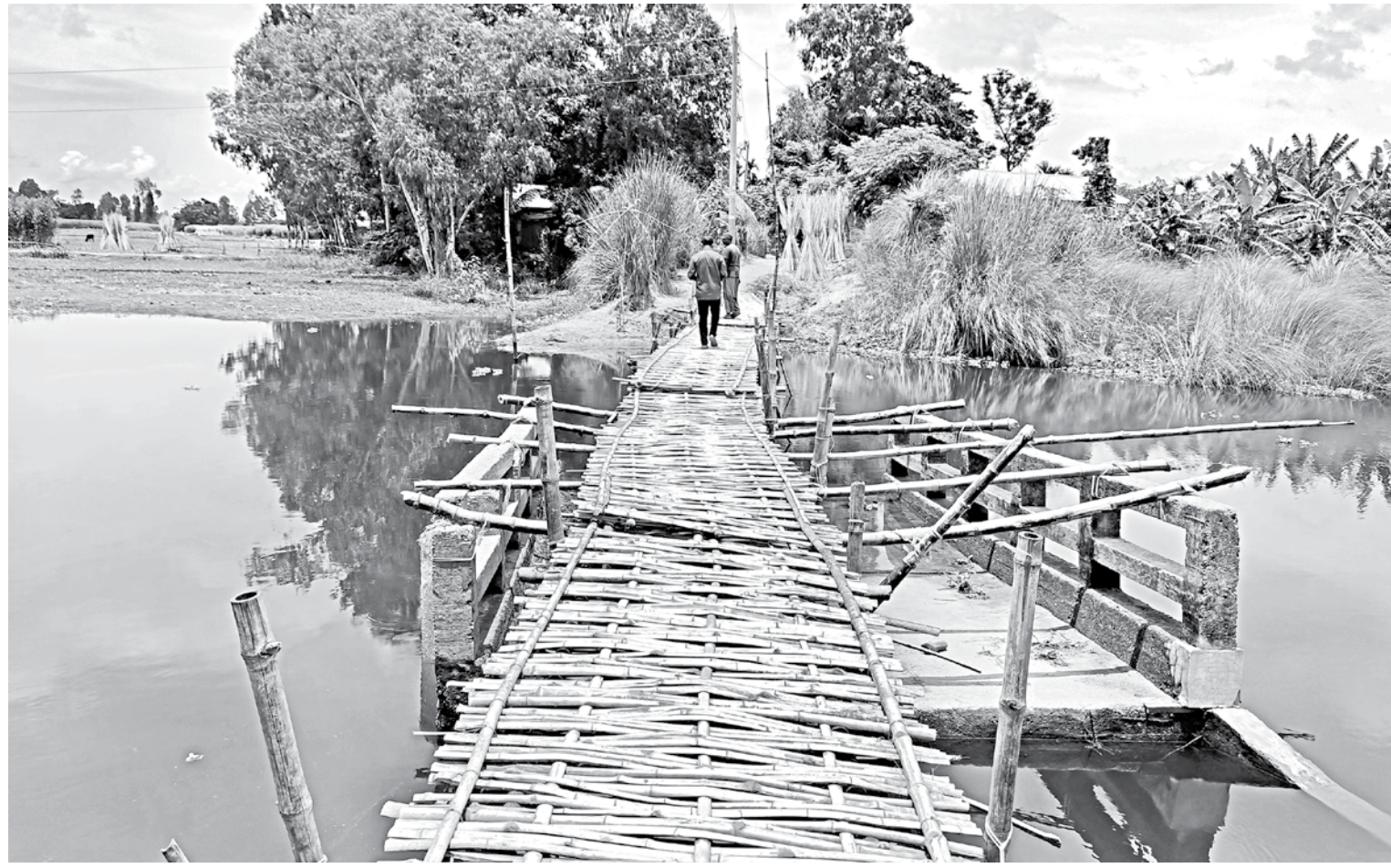
A makeshift bamboo bridge built by villagers over a damaged concrete bridge in Char Gaytapara of Kurigram's Roumari upazila.
