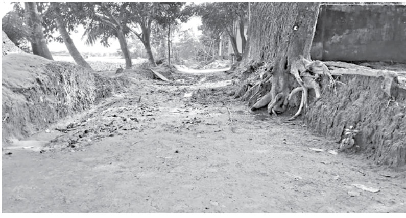
The Nolandaid to Nasirakanda road was dug up three years for development works. Today, it is in such bad condition that no vehicle can run on it, including rickshaws.
