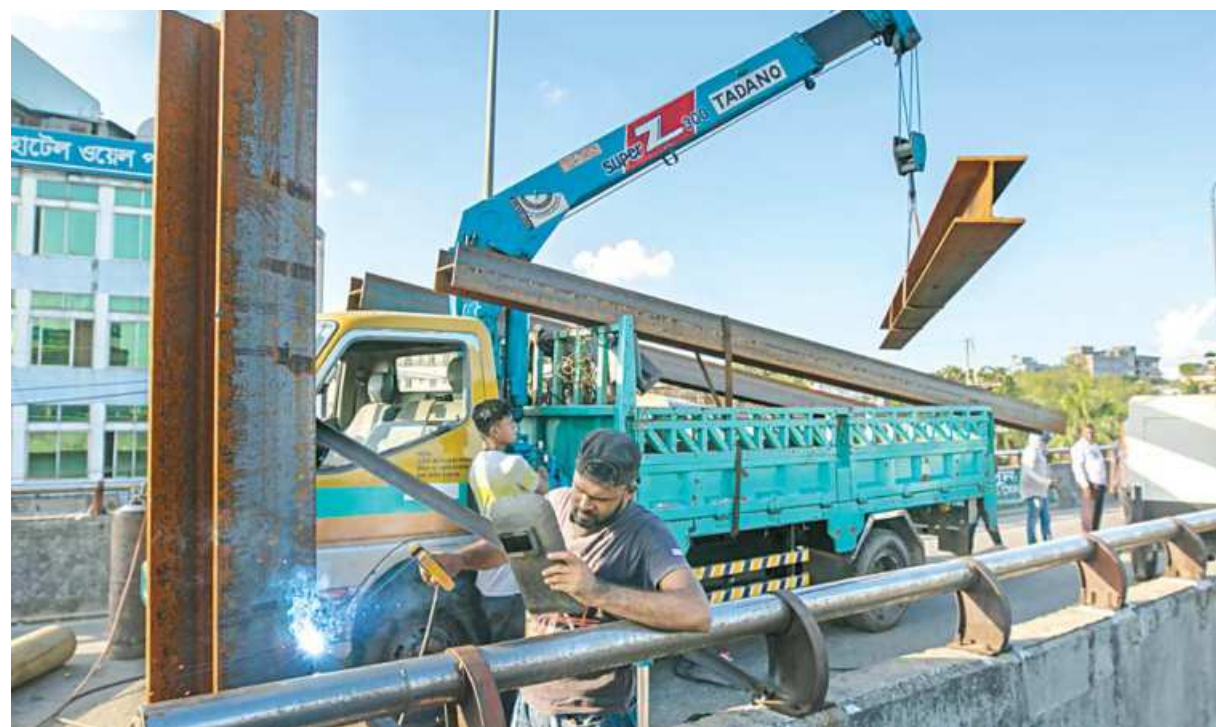
Closed due to fears over cracks emerging on its surface, the port city's MA Mannan Flyover's Kalurghat-ramp is getting height barriers installed to control movement of heavy vehicles. This photo was taken from Bahaddarhat area yesterday.
