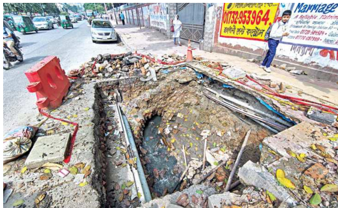
Dhaka South City Corporation authorities dug this hole on the capital's Mirpur Road close to Dhanmondi Govt Boys' High School for the renovation of a drain. This has been in this state for nearly two weeks, shrinking the road space and causing inconvenience to pedestrians, including the students of the school. The photo was taken yesterday.
