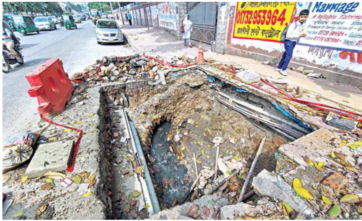
Dhaka South City Corporation authorities dug this hole on the capital's Mirpur Road close to Dhanmondi Govt Boys' High School for the renovation of a drain. This has been in this state for nearly two weeks, shrinking the road space and causing inconvenience to pedestrians, including the students of the school. The photo was taken yesterday.
