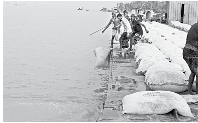
As part of a project launched recently to contain erosion of the Tentulia river, workers of BWDB dump geotextile bags in Dhulia area under Patuakhali's Baufal upazila. PHOTO: SOHRAB HOSSAIN
