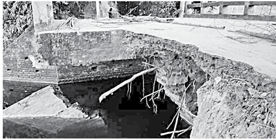
Part of a bridge on Korail-Hilora-Adabari road in Mohera Union Parishad under Mirzapur upazila of Tangail has recently collapsed, snapping road communication in the area and causing suffering to the commuters. PHOTO: MIRZA SHAKIL
