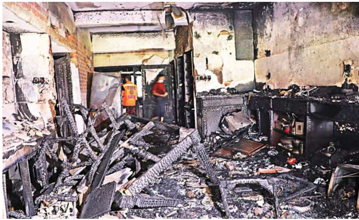
A fire fighter inspects the damage caused by a fire that broke out at this residence in the capital's Gulshan yesterday. Four people, including a couple and their two-year-old son, suffered burn injuries. The fire broke out around 11:30am and eight firefighting units doused it around 1:15pm.
