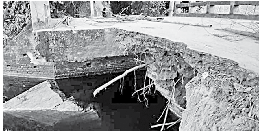
Part of a bridge on Korail-Hilora-Adabari road in Mohera Union Parishad under Mirzapur upazila of Tangail has recently collapsed, snapping road communication in the area and causing suffering to the commuters. PHOTO: MIRZA SHAKIL
