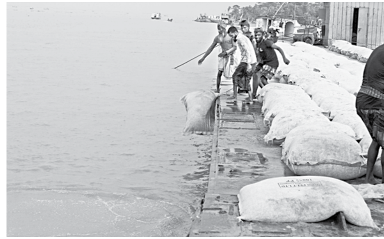
As part of a project launched recently to contain erosion of the Tentulia river, workers of BWDB dump geotextile bags in Dhulia area under Patuakhali's Baufal upazila. PHOTO: SOHRAB HOSSAIN
