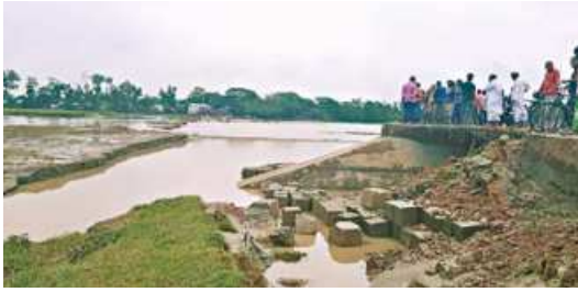
People standing on the remaining part of flood by-pass of the Teesta barrage in Lalmonirhat yesterday after it got damaged by a flash flood the day before.
