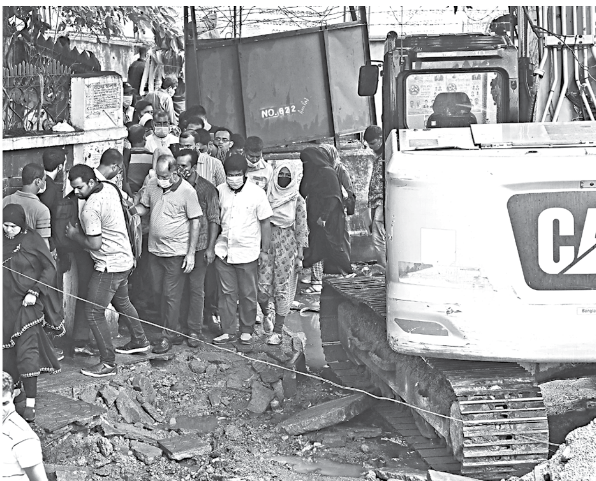
Near Shahbagh's Bangabandhu Sheikh Mujib Medical University, parts of the footpath is obstructed with materials for development works. As a result, pedestrians have to walk through the narrowed and broken pavement, squeezing into single lines to pass the area. One slip, and the result could be an accident. This photo was taken yesterday.
